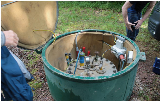
Figure 33: One of the older wells, of which there are 4. These wells used to extract water from both the 3rd and the 4th aquifers. Later on, eight new wells were constructed (figure 34), due to a needed increase in extraction capacity. The older wells continued to extract from only one of the two aquifers.
